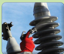
Importance of hydrophobicity and related tests in the electrical insulation industry
